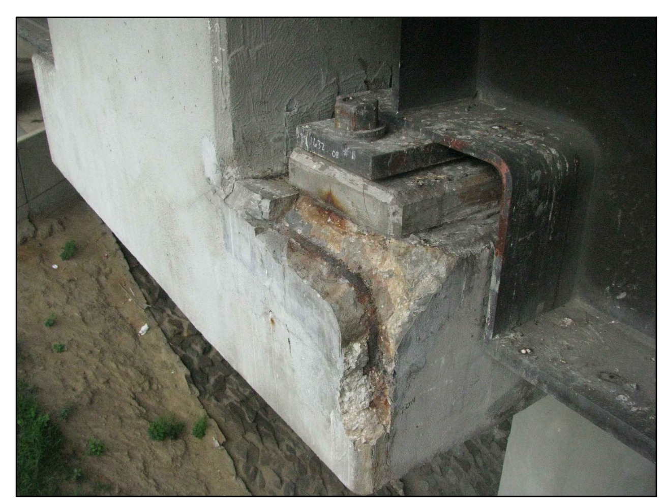
3 TYPICAL PIER CAP SPALL AT BEAM BEARING B04-S-914
